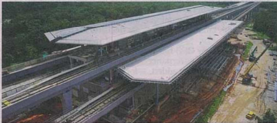
Filepic of the Kwasa Damansara MRT station under construction. SCSB is tendering for job packages from the SSP line, and AZSB had submitted a tender for the SSP line.
